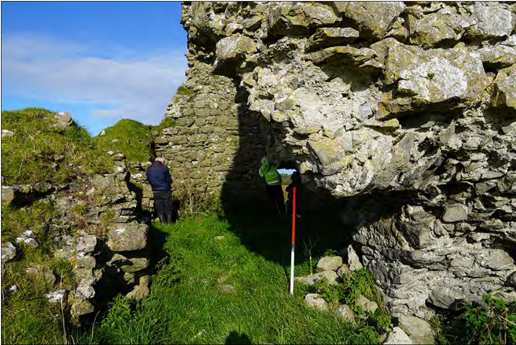
Figure 2.43. Window 1, partially collapsed, from SE. Only the N side of the embrasure survives. (F. Coyne).
