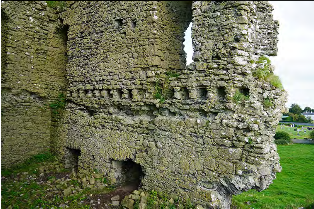
Figure 2.52. The slots for timber beams (likely oak) on the inner face of the SE wall, from W (F. Coyne).
