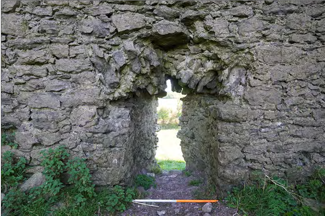
Figure 2.47. Window 4, note slot for timber lintel and robbed out flat arch, from SW (F. Coyne).
