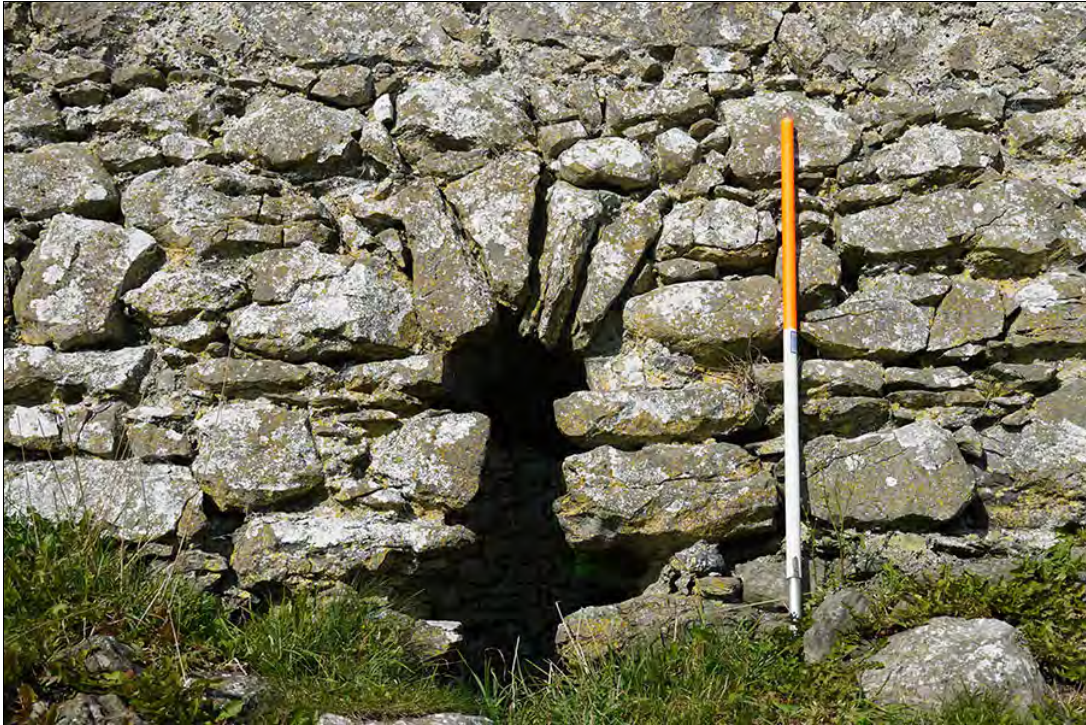
Figure 2.45. Window 2, mostly intact external window with complete arch, although rudimentary arch, from SE (F. Coyne). The light is approximately 0.2m wide.
