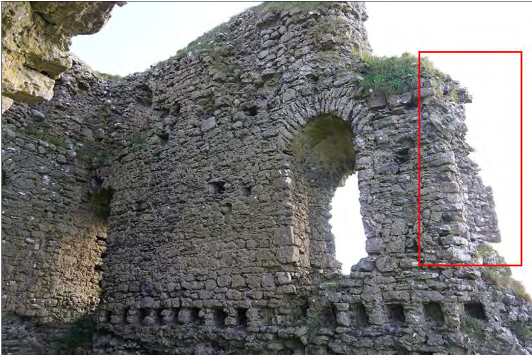
Figure 2.53. Window 1.1, only left side of embrasure remaining, from NW (F. Coyne).
