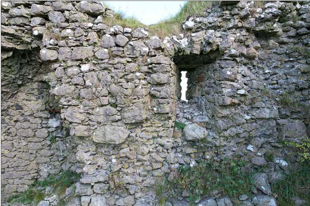
Figure 2.65. Loop in stairwell on 2 nd floor, window ope 2.2 on right, from SW
