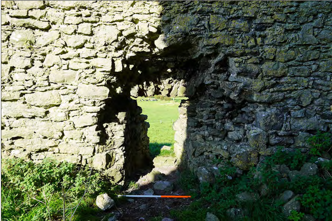
Figure 2.49. Window 6, note robbed out flat arch and jambs, from SW (F. Coyne).
