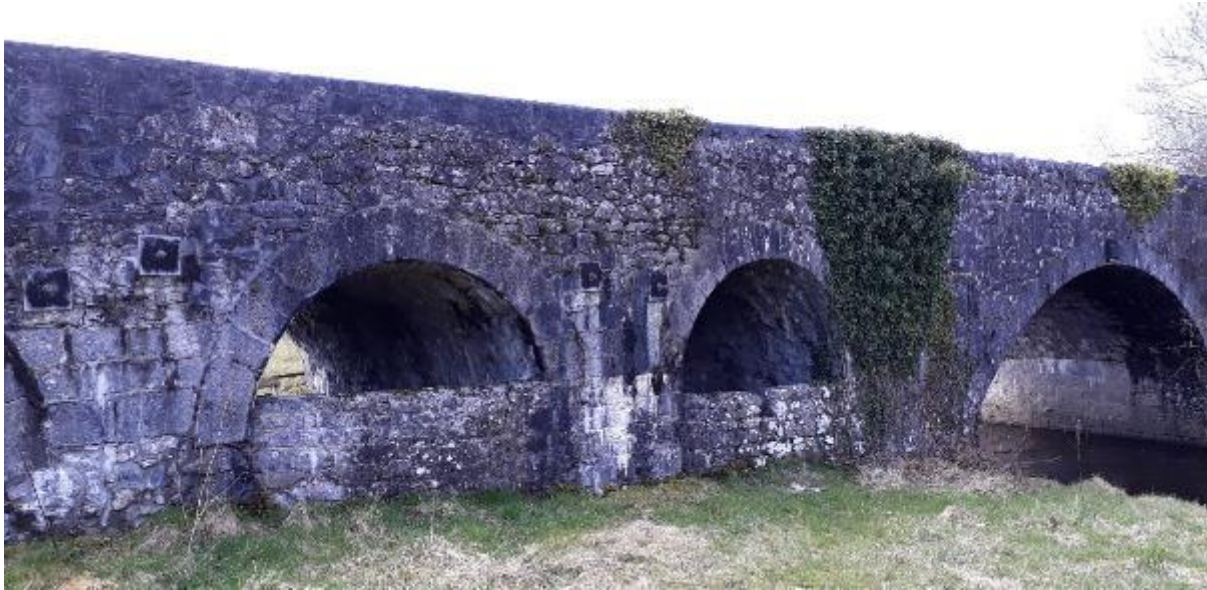
Photograph 116: Pallas bridge with blocked arches and one functioning arch.
