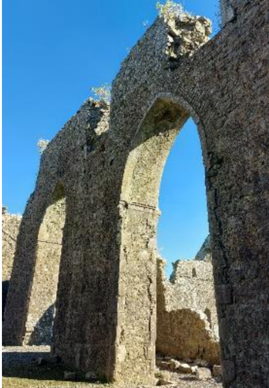
Photograph 11: Arcade of arches and piers separating the nave from the aisle with clerestory window openings above.
