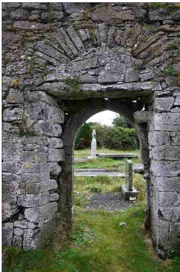
Figure 2.44. Internal view of church door, from N. Note infill and cracked lintel over door.
