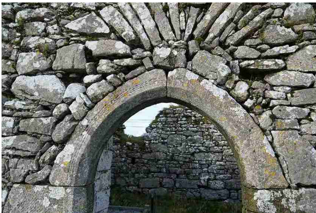
Figure 2.43. Detail of hyphenated decoration and sparrow pecking on S door, from S.
