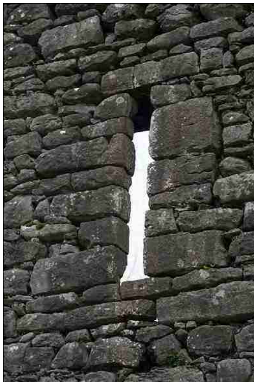
Figure 2.49. Detail of 15 th century window (external), from W. Note cracked lintel.
