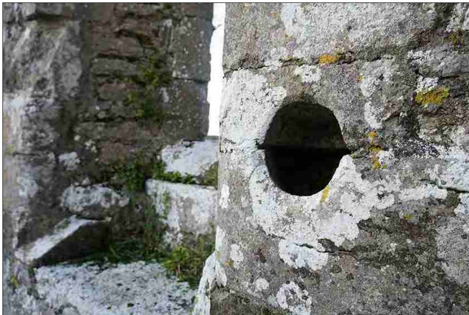
Figure 2.35. Hole on E side of N window, from SE.
