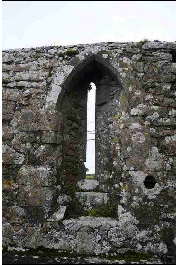
Figure 2.34. Window in N wall, from S. Note hole to right of window.
