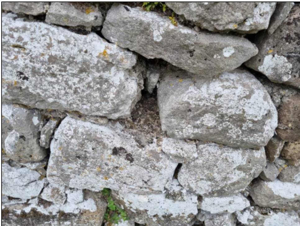
Plate 15: Detail of mortar missing on the outside face of the south wall.
