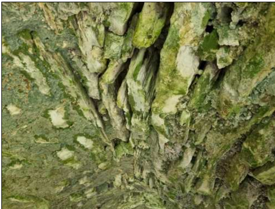
Plate 9: This photograph shows a view of the eroded hard lime mortar pointing to the stone voussoirs in the fifteenth-century vault ceiling.
