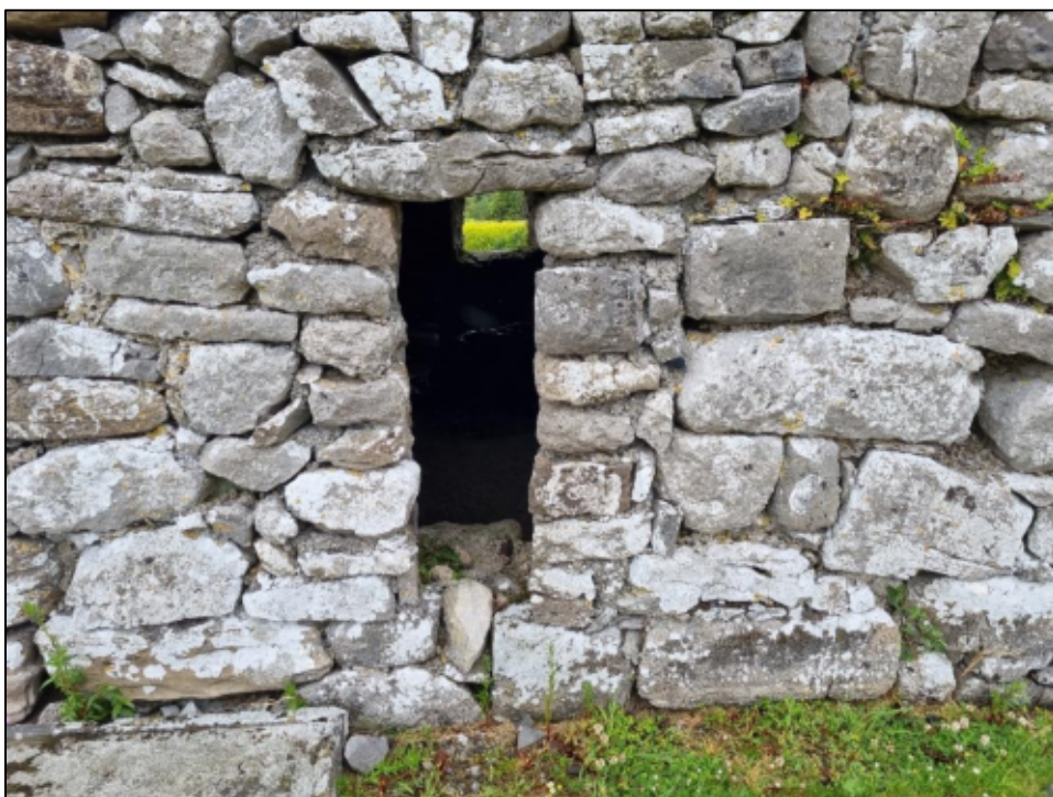
Plate 16: Notice the poor-quality bonding of masonry showing window alteration in the nineteenth century on the south wall (twelfth–thirteenth century).
