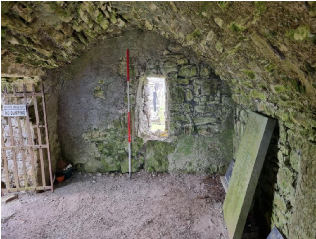
Plate 13: Further view of the south wall (twelfth–thirteenth century) showing soft lime plaster which probably dates from the nineteenth century.
