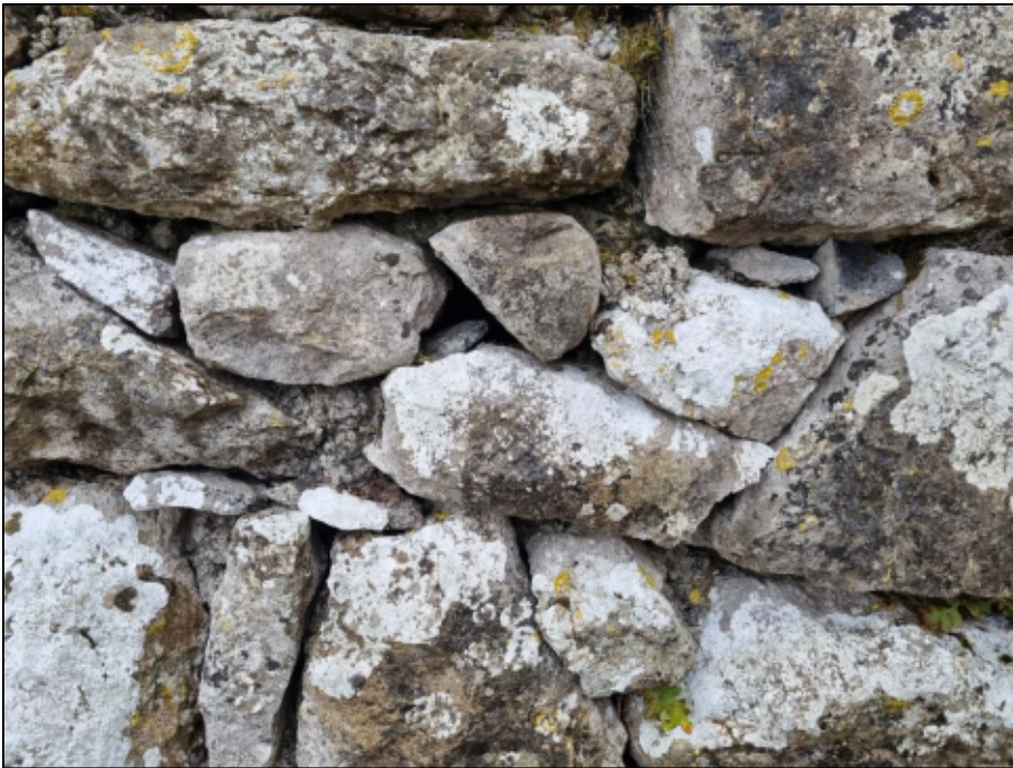
Plate 6: Detail of the decayed pointing but with bedding mortar present behind, some recent poor-quality cement pointing to be removed.
