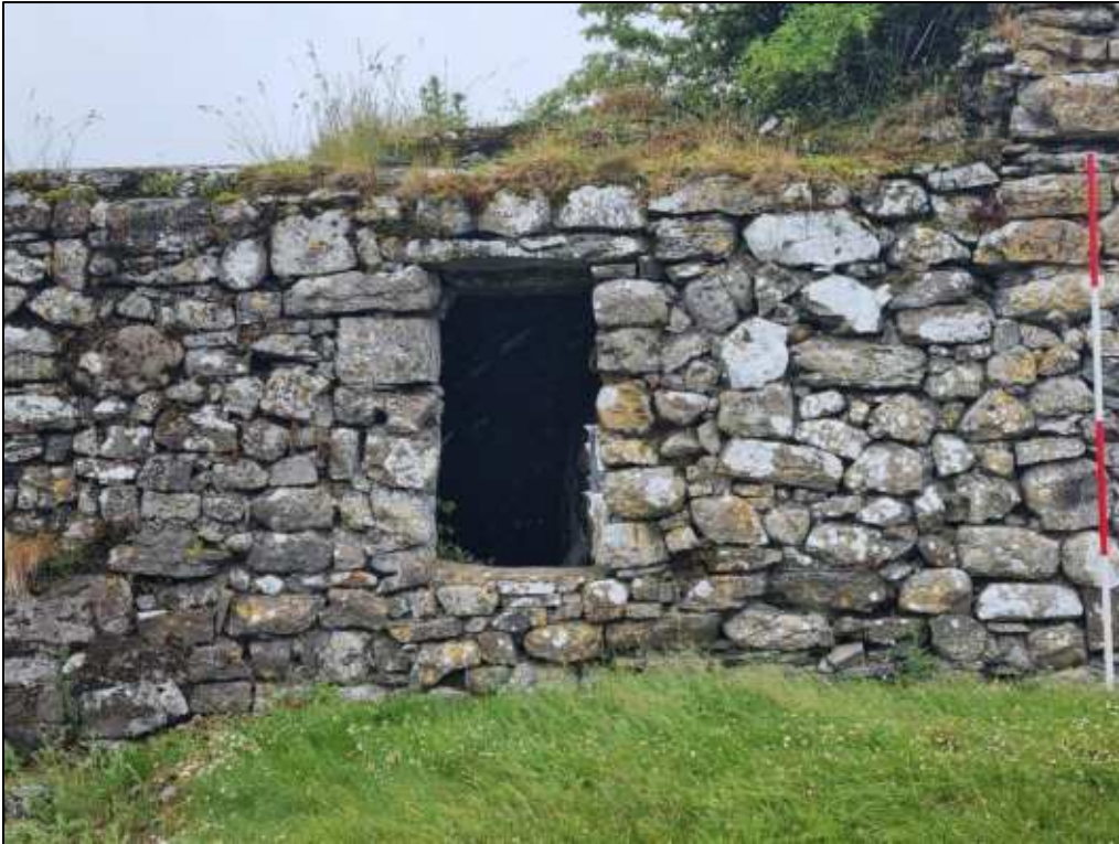
Plate 19: Again, the poorer quality alteration to window in the north wall of the vault. To the left of this another vertical line shows the area of reconstruction (suggested eighteenth-century) in mud mortar.
