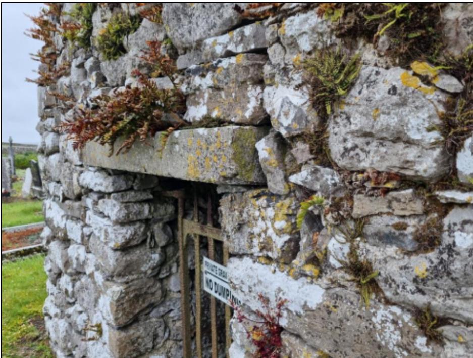
Plate 7: The lintel over the door to the vault appears to be a more recent replacement. It is proposed to leave this in situ .
