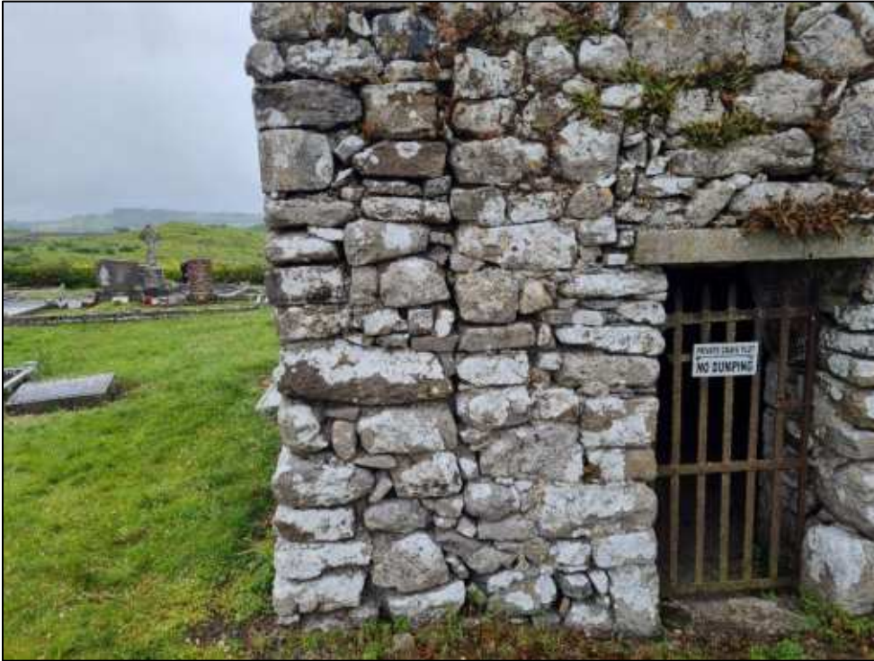
Plate 4: View of the junction between the south wall and the wall enclosing the vault.
