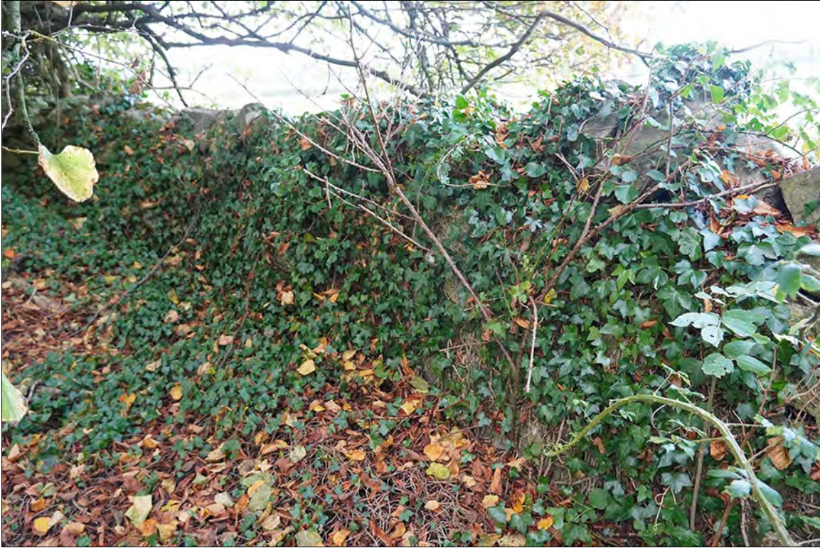
Figure 2.45. Overgrown graveyard wall at N, from SE (F. Coyne).
