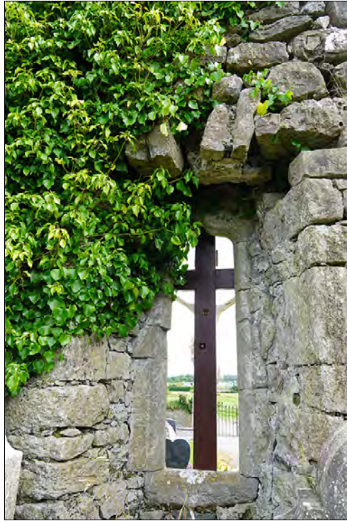
Figure 2.46. Internal view of E window, from W. Note ivy and collapsing arch (F Coyne).
