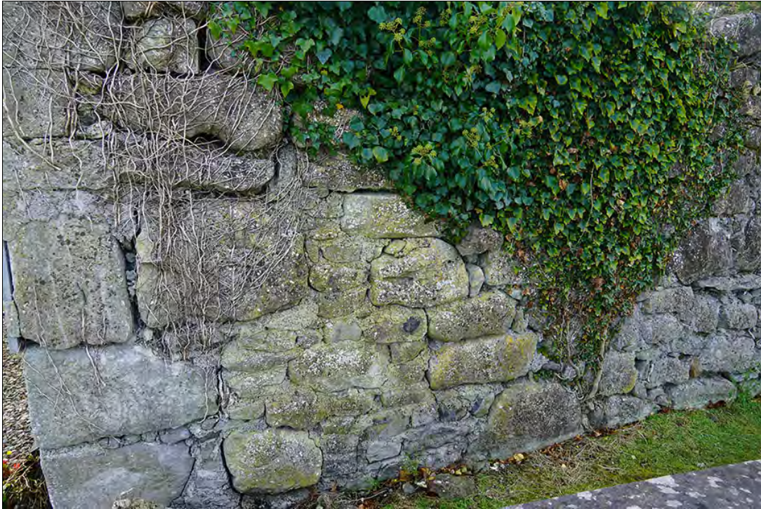
Figure 2.64. Structural crack in N wall externally at NE corner, from N (F. Coyne).
