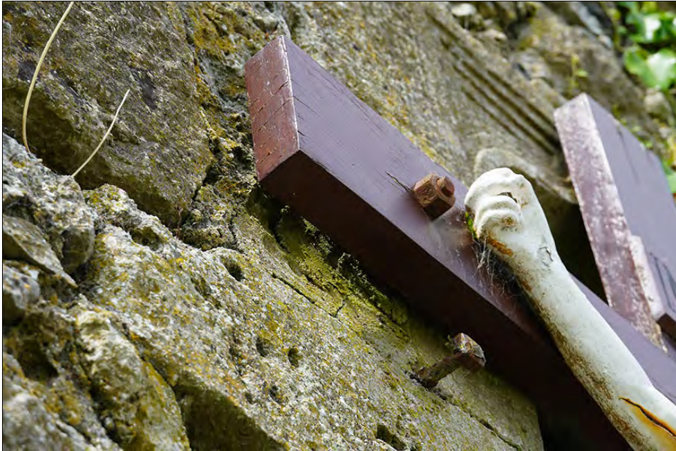
Figure 2.44. Detail of modern bolts on the external face E window, from SE. These were inserted into the bedding joints. (F Coyne).
