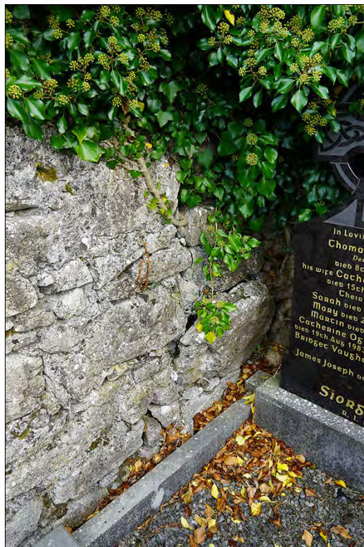
Figure 2.65. Structural crack in N wall internally at NE corner, from SW (F. Coyne).
