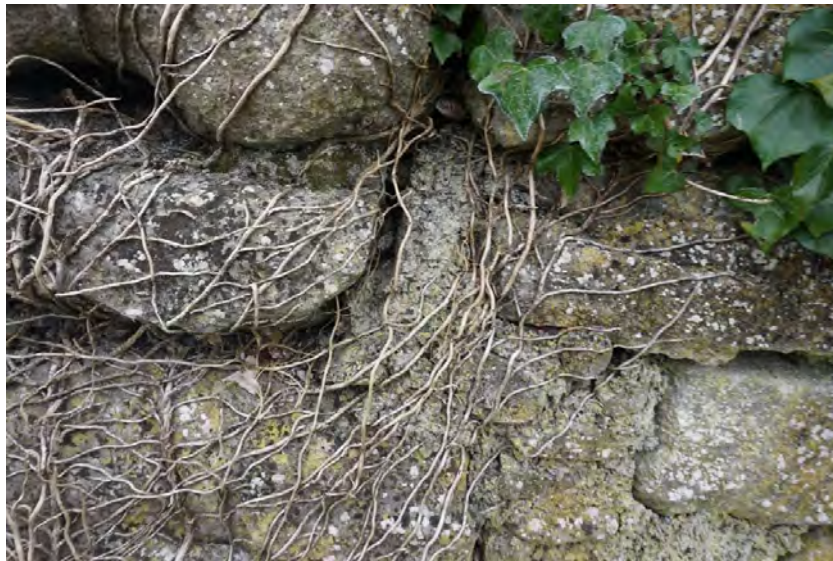
Photograph 3 Detail from the northern elevation demonstrating the mortar used in the remedial works. Note large aggregates of the sharp sand.
