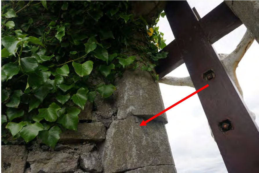
Photograph 17 View of the window jamb stones. Note shear damage to the lower unit from the pressure of the lean of the wall.
