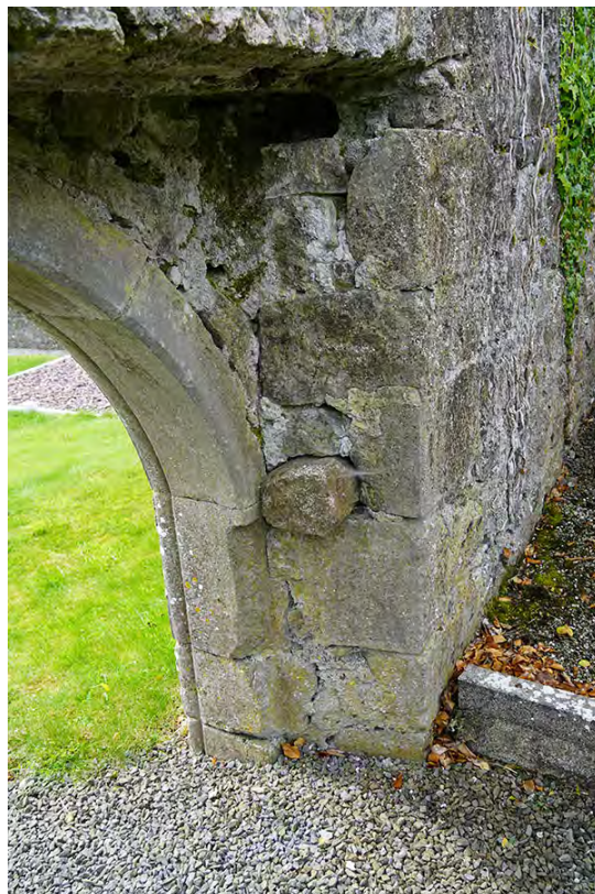
Figure 2.59. Drawbar socket on internal side of door, from NE. Note loose stone placed in socket (F. Coyne).
