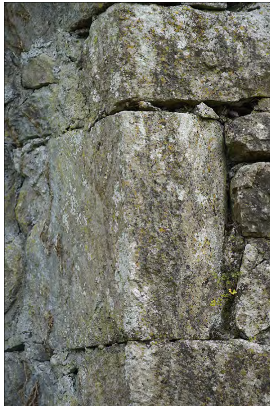
Figure 2.47. Reused chamfered stone internally on E window. This stone contains 12 th /13 th century diagonal tooling. Note ivy and collapsing arch (F Coyne).
