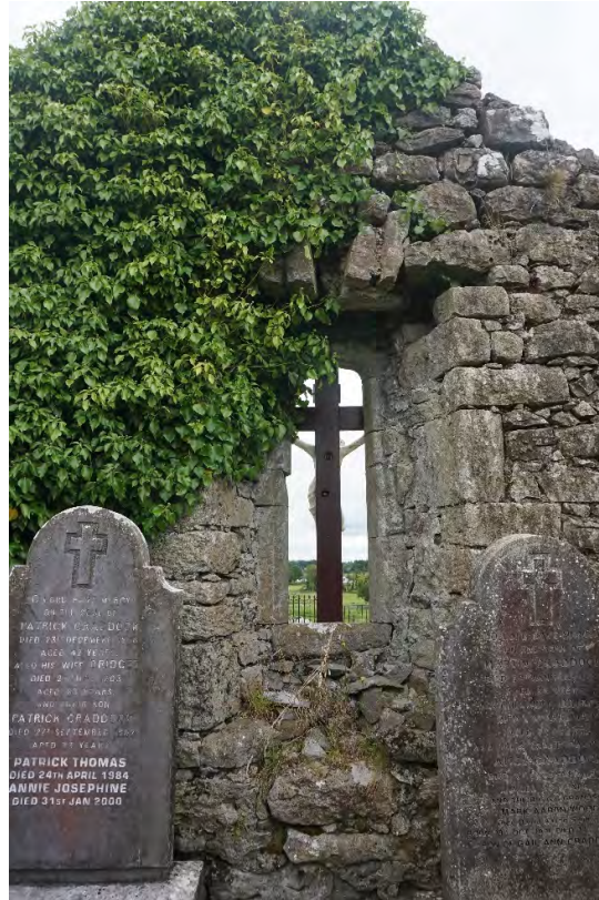
Photograph 15. Internal view of the eastern gable opening. Note missing voussoirs.
