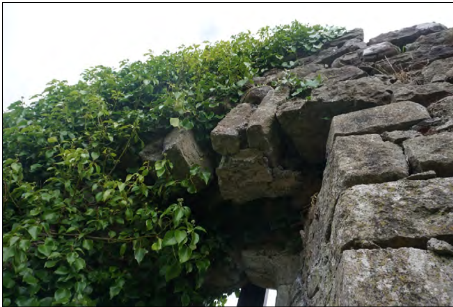
Photograph 16. Bottom-up view of the internal arch soffit. Units dangling dangerously.
