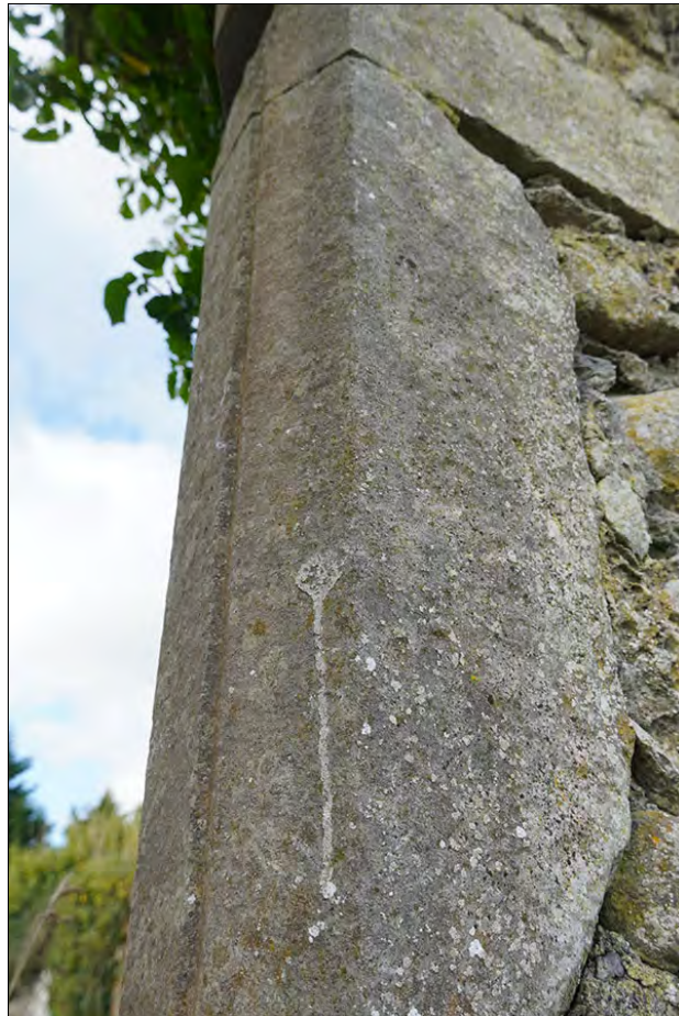
Figure 2.45. Detail of rebate for glazing on the external face E window, from E (F Coyne).
