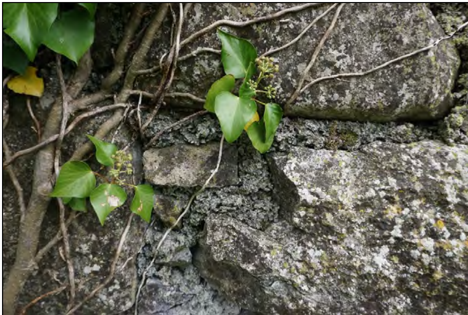
Photograph 7 Detail from the western wall. Note cementitious mortar and pinning stone reinstated.
