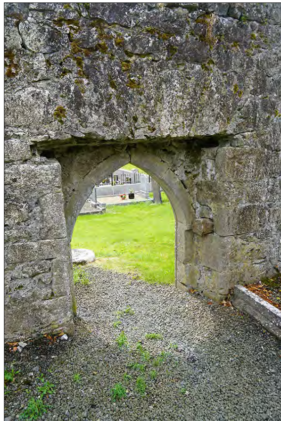
Figure 2.57. Internal view of door, from S. Note void for timber lintel (F. Coyne).
