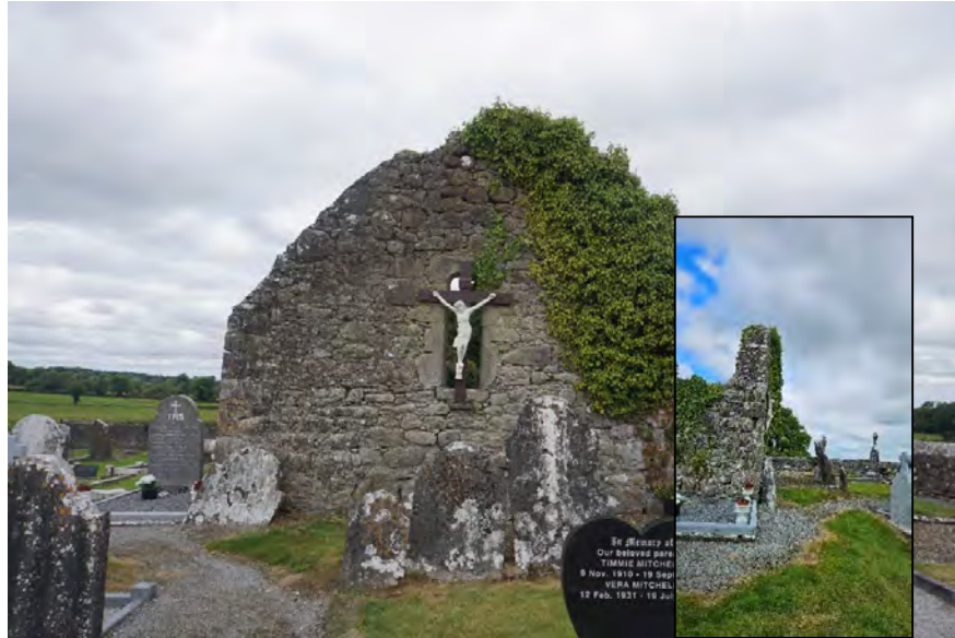
Photograph 13 Eastern elevation view. Inset, side plane view, note lean of the wall outwards.
