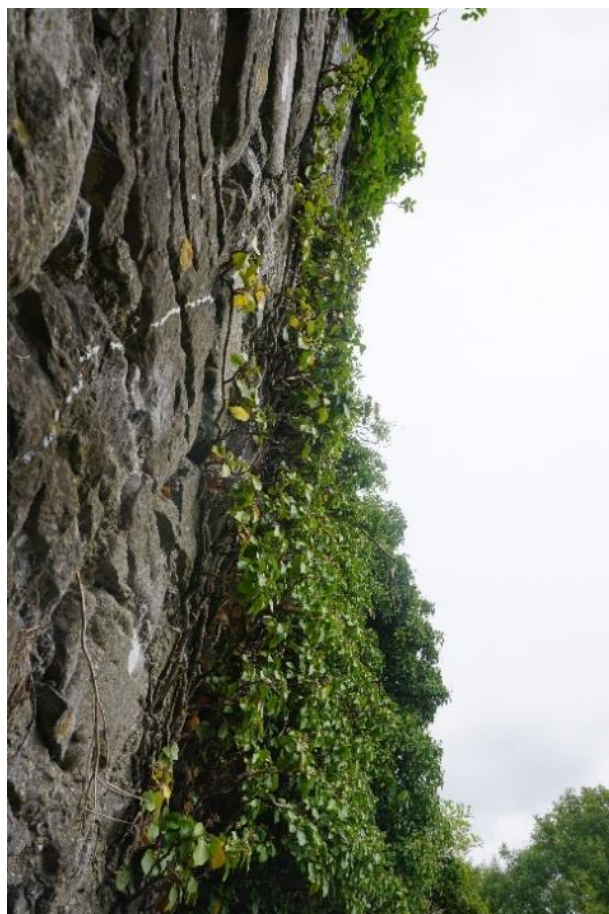
Photograph 3 View of the upper western gable end from inside the footprint of the building ruin.
