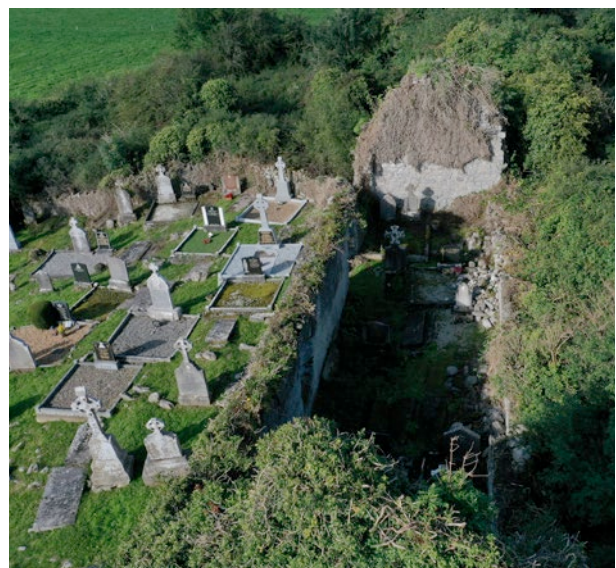
Aerial view looking West, showing ivy growth at West gable
