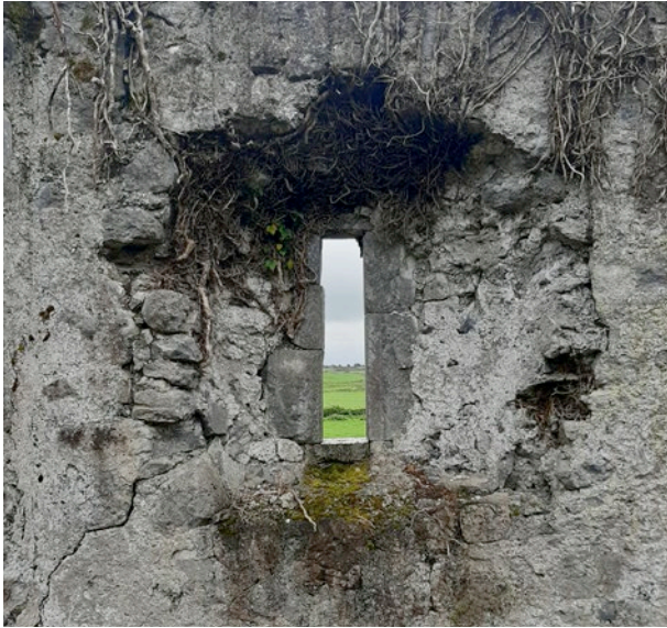
Internal view of the window at the East end of the extended South wall
