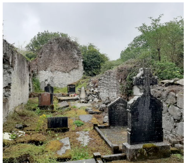
General interior view looking West, showing condition of North wall on the right
