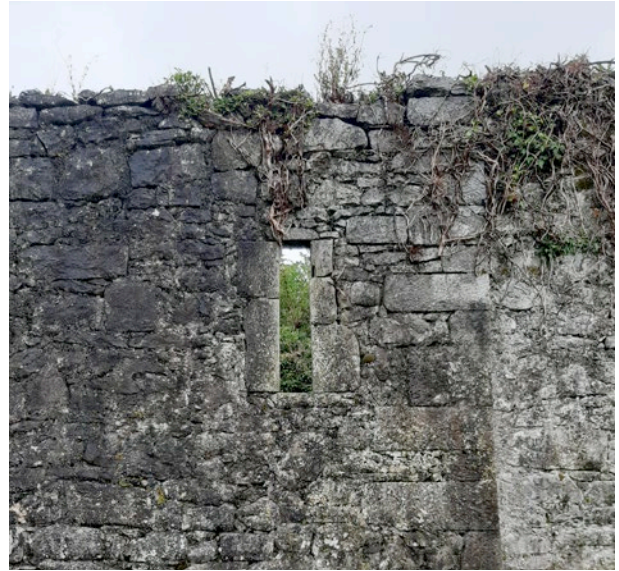
External view of the window at the East end of the extended South wall
