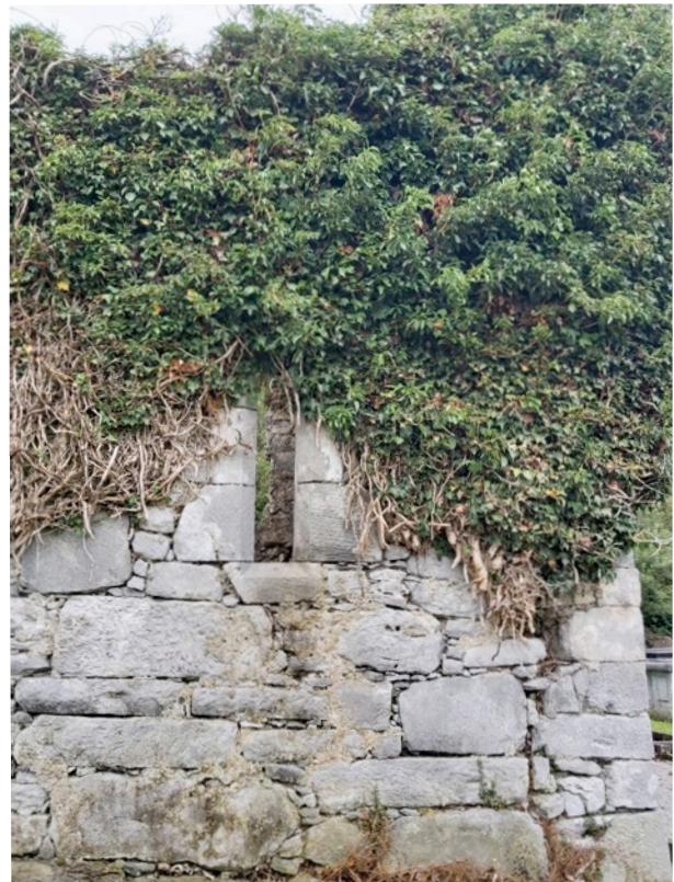
View of window on Eastern end of South wall, showing ivy growth
