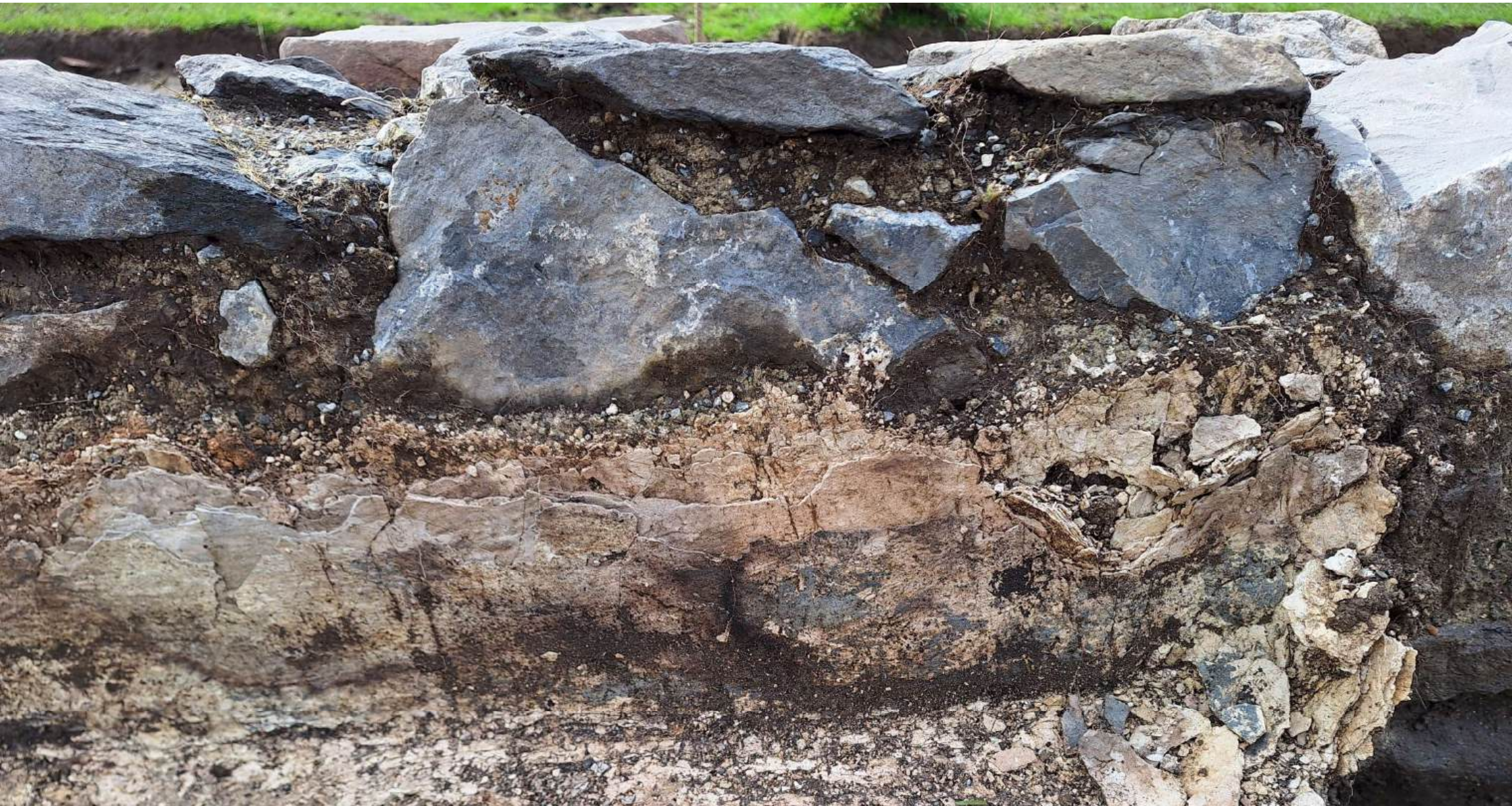
Hugh Carey ancestral house: detail of lime render (internal) and rubble wall construction
