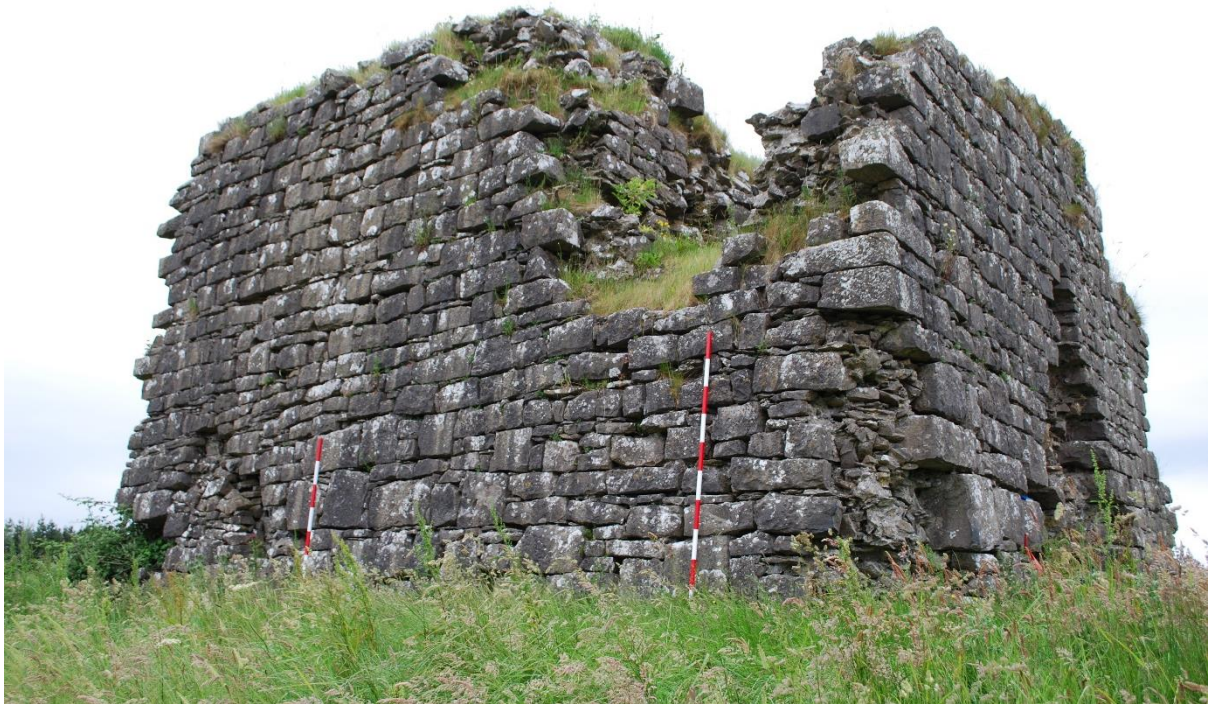
Fig. 9. The west wall of the tower house with breach indicating position of former window embrasure on first floor above the vault.
