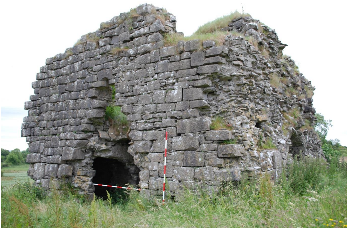
Fig. 10. South wall showing breached entrance, mezzanine chamber window and tiny loop on stairwell in southeast corner.
