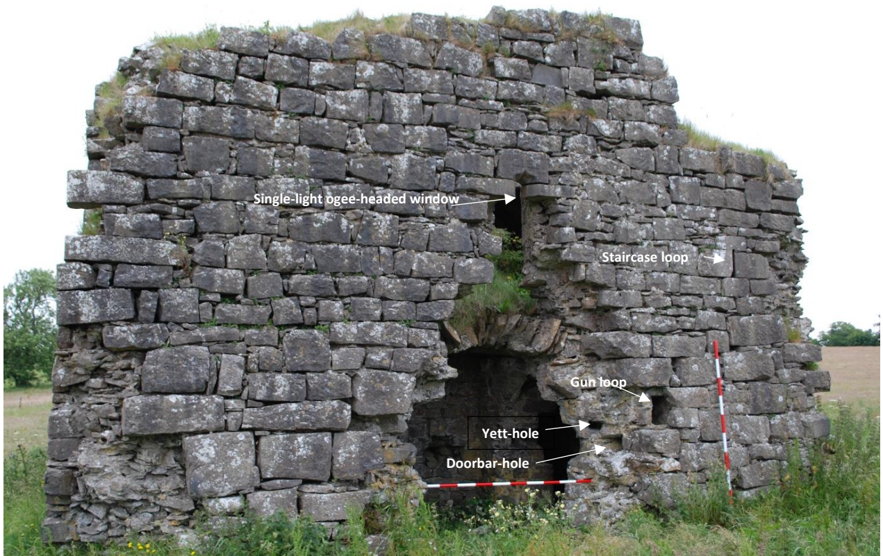
Fig. 12. The south wall showing the breached entrance, gun-loop to the right, a single-light ogee-headed window on the first floor above the doorway and a narrow round-headed loop lighting the staircase.
