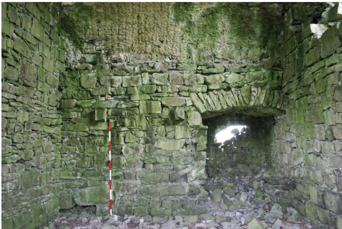
Fig. 26 West wall with blocked window and fragmentary corbels for mezzanine floor beams.
