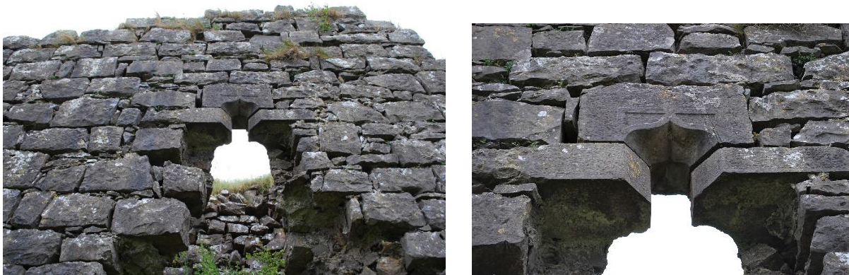
Fig. 29 Remains of ogee-headed window in south wall lighting the mezzanine chamber on the south side of the cross-wall.
