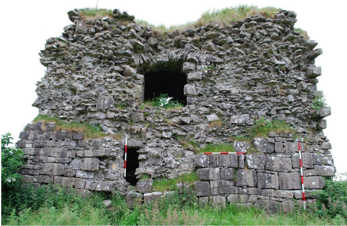
Fig. 7. North wall with extensively robbed out masonry above ground floor level.
