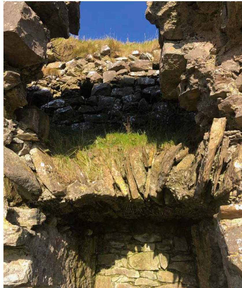
52. Detail of exposed and unstable floor and walls over entrance.
