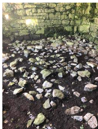
34. Loose stone to floor.
