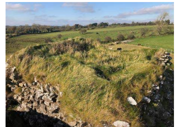
38. View looking north over main vault showing grass covering and eroded wall tops.
