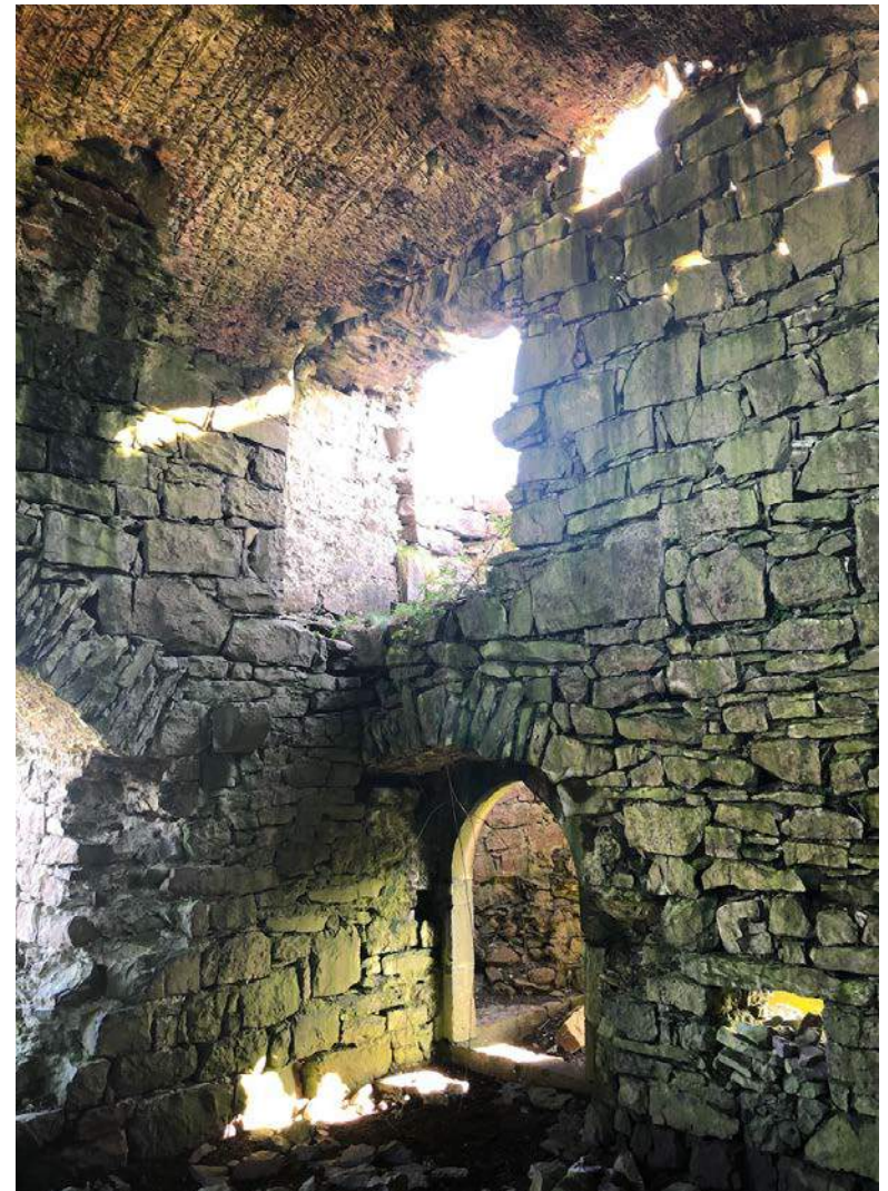
35. View of subdividing wall to main chamber. Note large voids to stonework at high level, corbels and squints.
