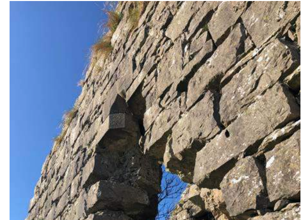
23. Detail of eroded ogee-window to south east face with extensive mortar loss to surrounding facing stone.
