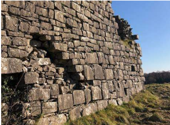
21. View of missing facing stone and drywall infill stone to window to south west face of tower house.
