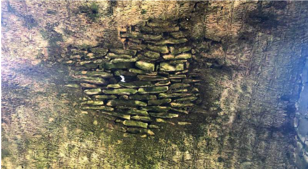
31. View of vault to main chamber, daylight visible to centre and extensive wash out of joints.
