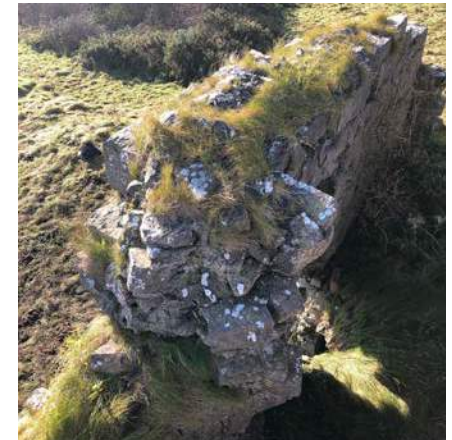
42. View of vulnerable masonry at top of stairs.
