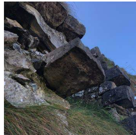
26. Detail of surviving facing stone at risk of collapse
